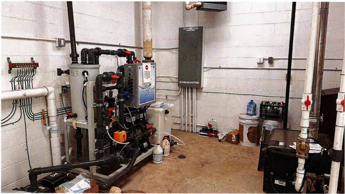
Pool Mechanical Room
