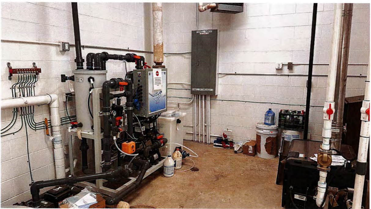
Pool Mechanical Room
