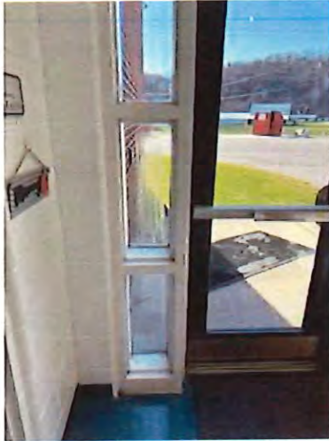
Photo 3: Window panels/frames needing replaced
