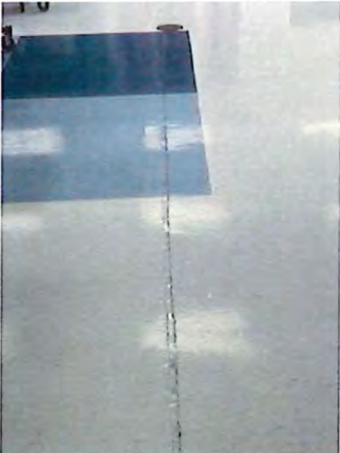
Photo 8: Cracked VCT – settling expansion joints
