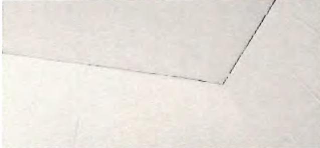
Photo 1: Drywall ceiling separating from walls.
