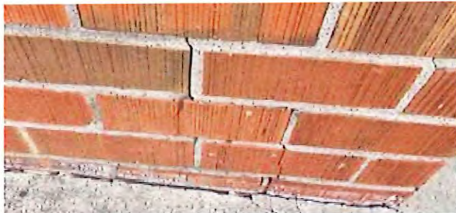
Photo 6: Cracked bricks/mortar separation, concrete opening to base of building
