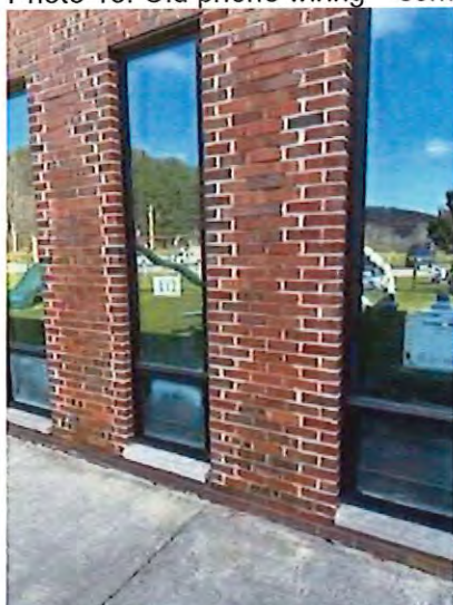
Photo 14: Exterior windows needing replaced and spalling brick
