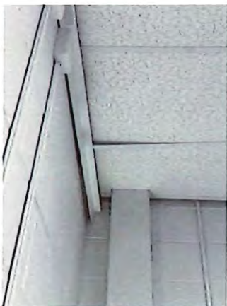
Photo 11: Multiple ceiling penetrations/Ceiling grid uneven
