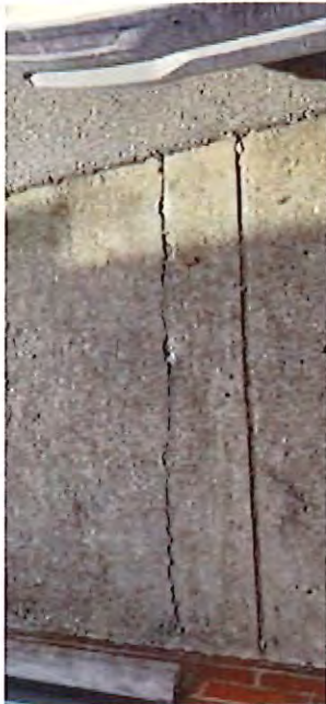
Photo 8: Cracked concrete sidewalks - settling
