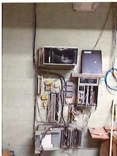
Photo 13: Old phone wiring – some parts of the system still utilized
