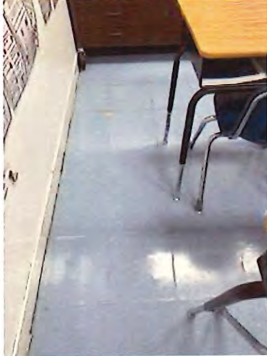
Photo 1: VCT floor tile with asbestos in the mastic.
