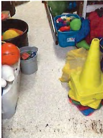
Photo 2: Vinyl flooring in gym storage with asbestos in the mastic.
