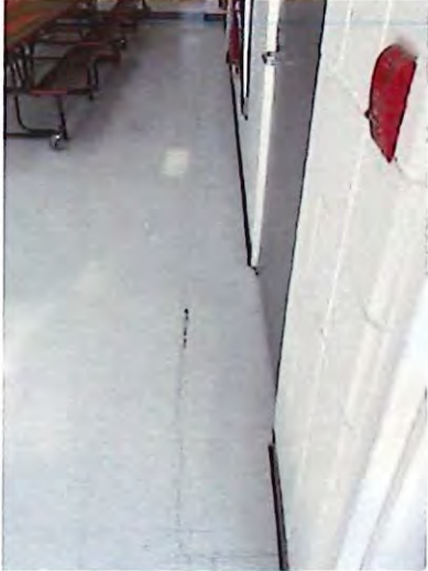
Photo 9: Cracked VCT – settling foundation
