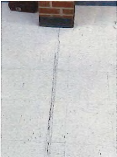
Photo 7: Cracked VCT – settling expansion joints
