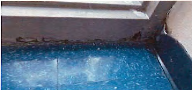
Photo 2: Rusting window frames.
