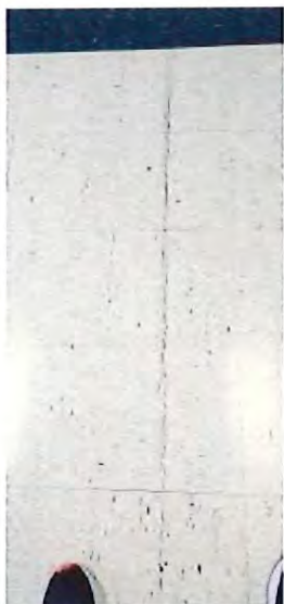
Photo 7: Cracked VCT – settling expansion joints
