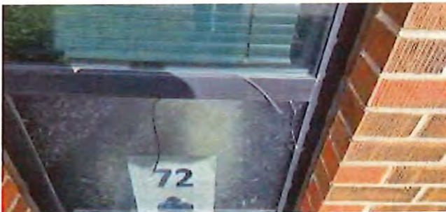
Photo 10: Exterior windows needing replaced and spalling
