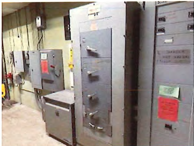
Photo 12: Electrical panel room – outdated panels
