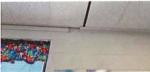
Photo 9: Multiple ceiling penetrations/Ceiling grid uneven
