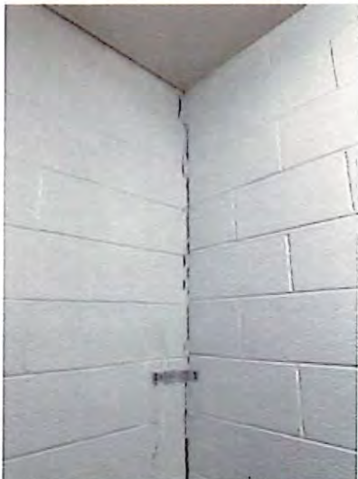
Photo 10: Cracking and wall separation
