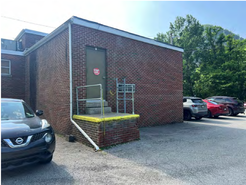
Loading dock at the 2006 addition with damaged brick from vehicles.
