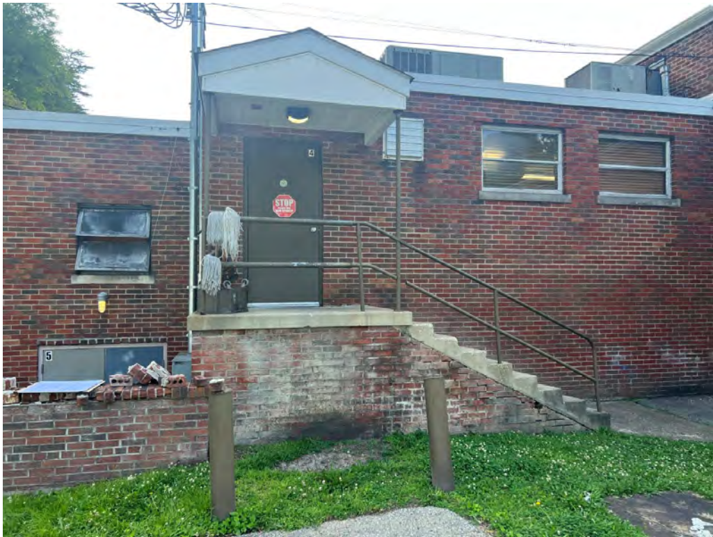
Elevated kitchen entrance showing signs of water infiltration and sprawling brick.
