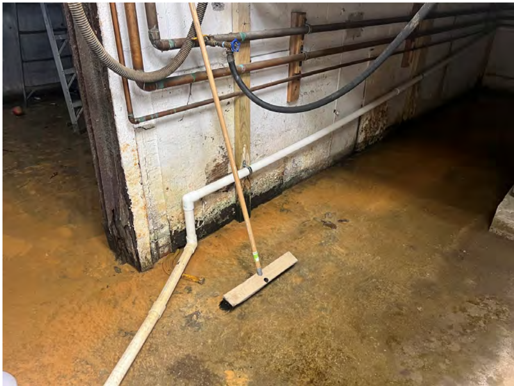
Standing water under the elevated janitorial space that serves as access to the crawl space.
