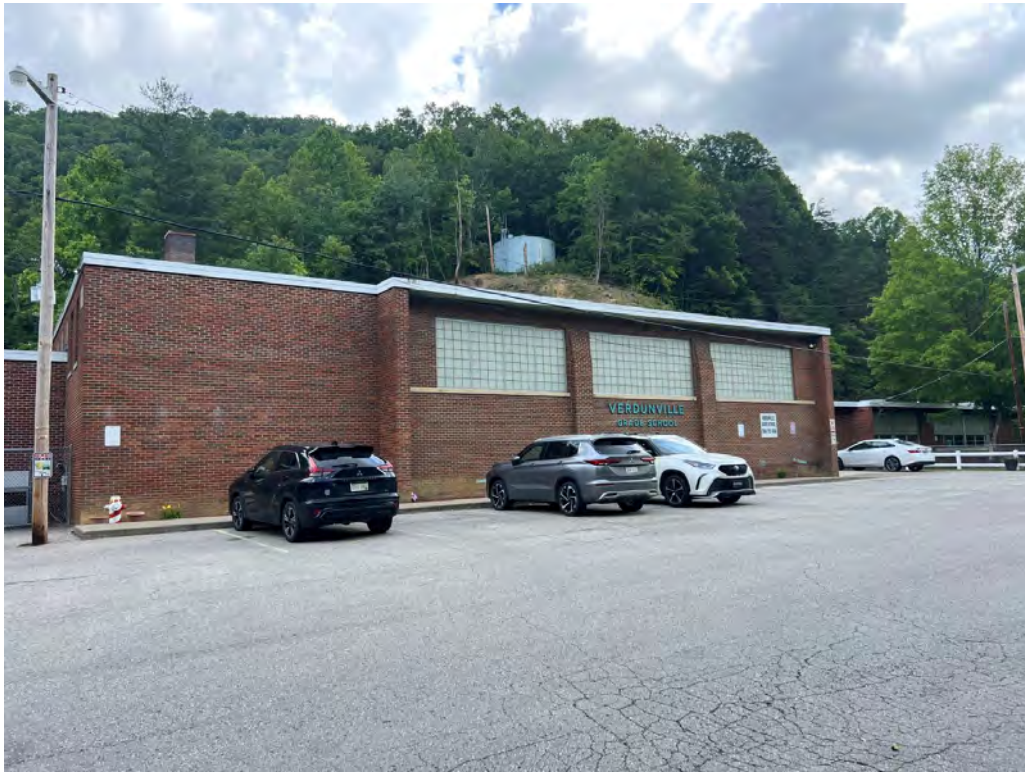
Front of the Multi-Purpose room. Signs of asphalt cracking are present in the lower section.
