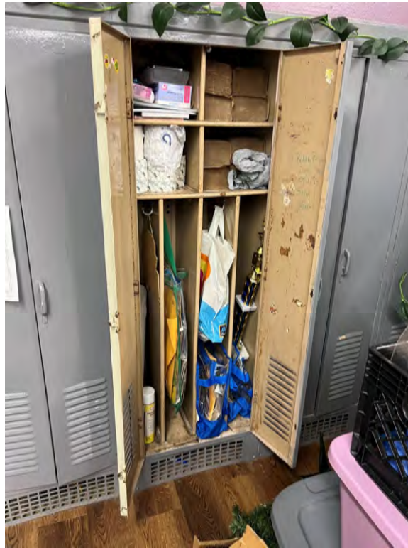
Existing lockers within classrooms. Lockers are in various conditions throughout the building.
